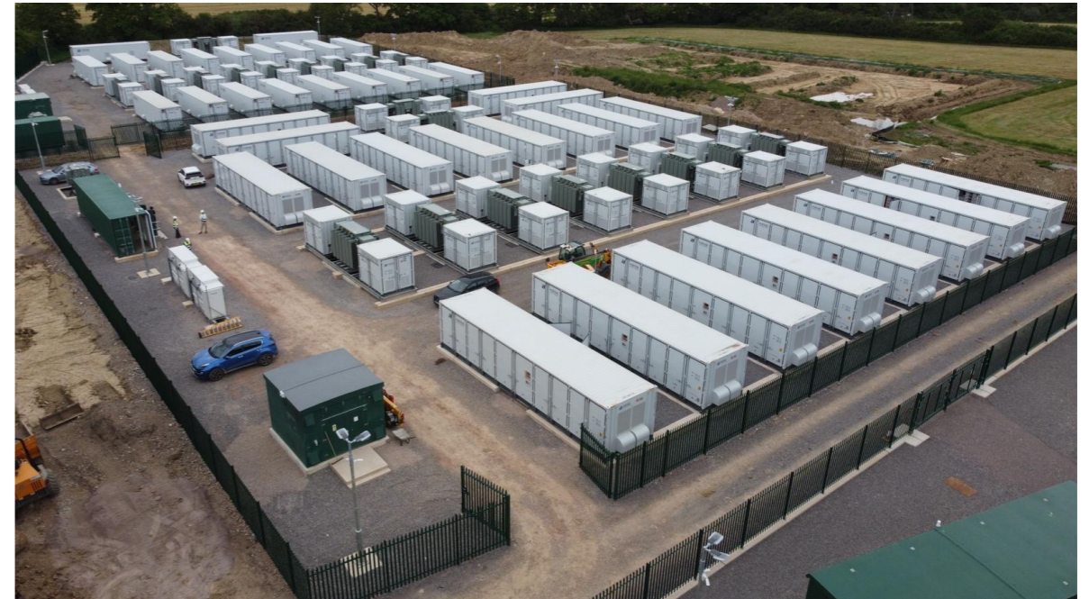
Diagram 1.3 Photograph of Minety battery storage; an example of a 100MW site
